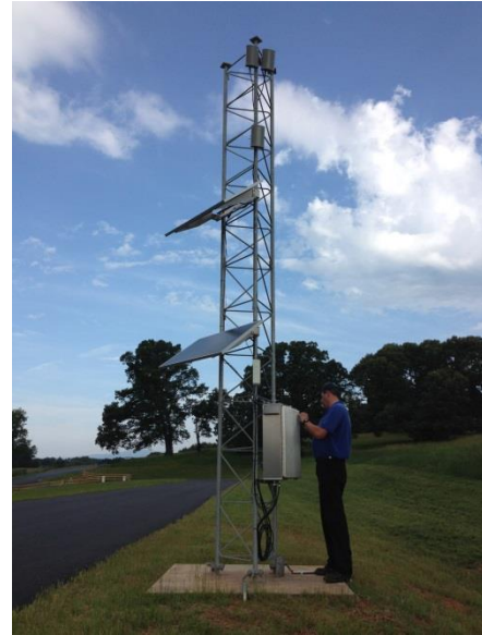
Figure 10: Permanent LocataLite Site
