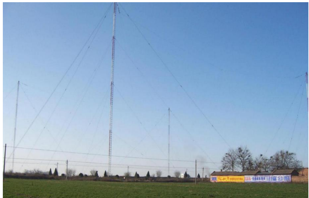
Figure 1. Four towers of the BPL antenna.
